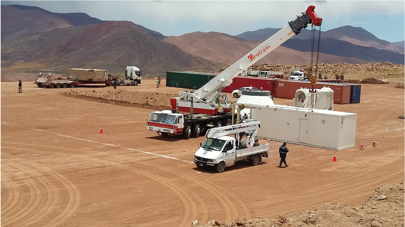
Figure 9. View of the installation of different components of LLAMA antenna in Alto Chorrillos . Credit: Fundación CAPACIT-AR and Instituto Geonorte, INENCO (CONICET).
